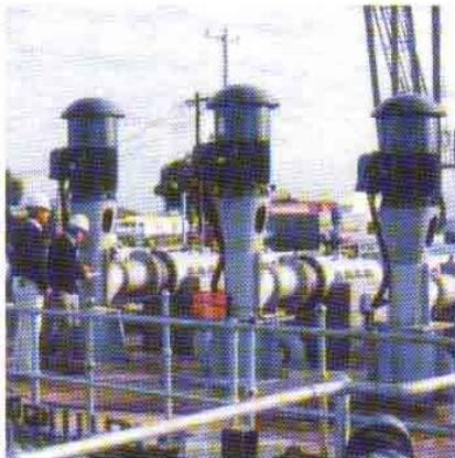
Five Batescrew 316L lineshaft Turbines installed for the NSW Public Works, irrigation pipeline rehabilitation. 100, 200, 300, 350, and 500 litres/second, 11 metre column length. Mildura, Victoria.
