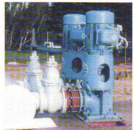
Town water supply, Wangaratta, Victoria. Batescrew 16HC pump delivers 200 litres/second. 14 metre head 45kw Motor continuous duty with 'stand-by' pump.
